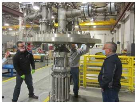
Liquid hydrogen fuel supply pump
