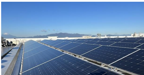
Solar power panels installed at Fujisawa Plant
