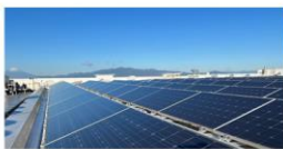
Solar power panels installed at Fujisawa Plant
