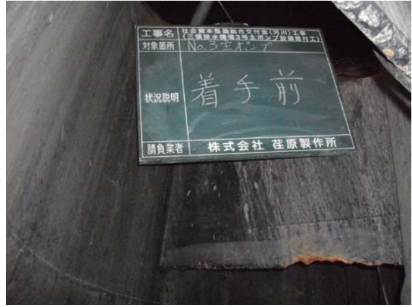
案内羽根壊食状況 Erosion at the suction vane
