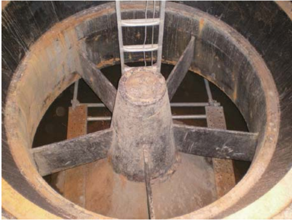
吸込側案内羽根全景 View of the suction vane
